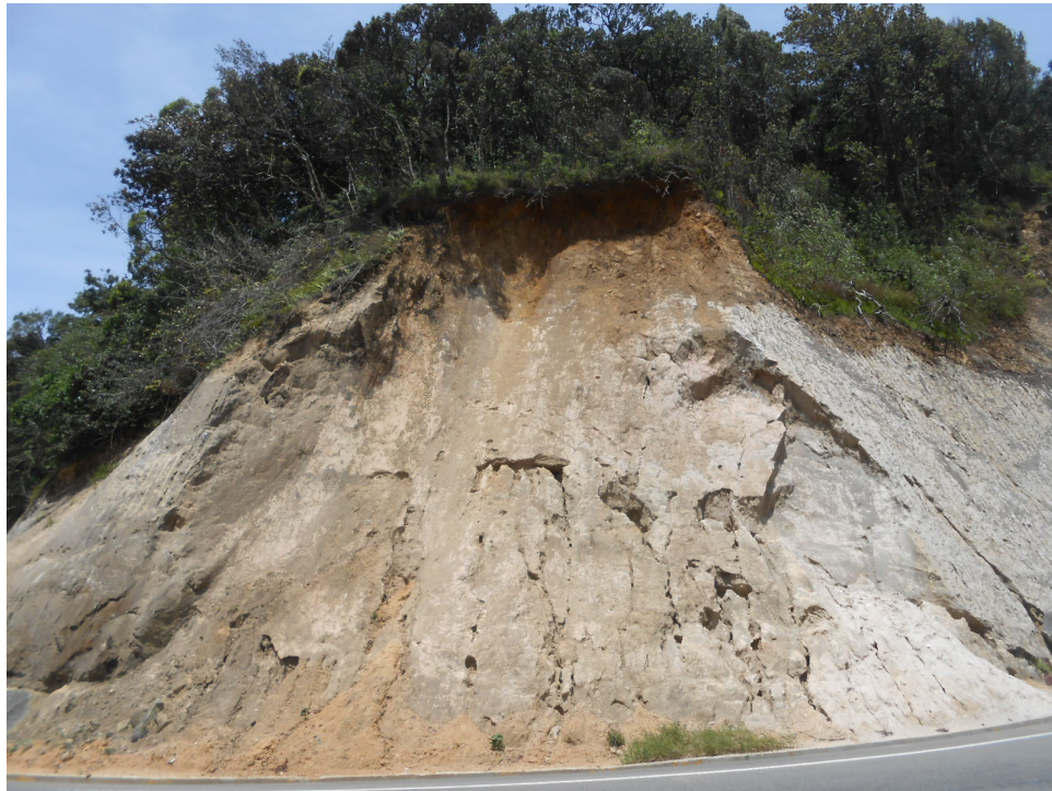
Figure 2: Cutting failure at Hakgala due to road cuts.
