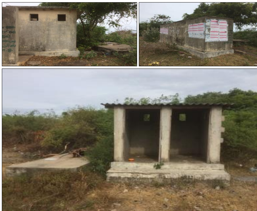
Figure 13. Condition of Public Toilets in the Underserved Settlements (Source: Field survey, 2020 & 2021)
